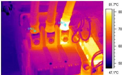
Figure 17.8 An infrared image of indoor electrical equipment (1).
